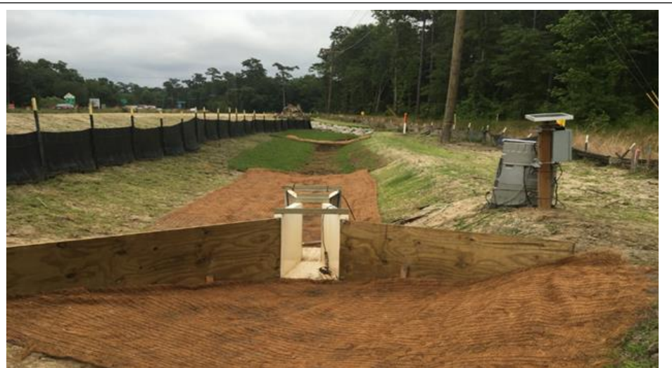
Linear BMP Monitoring Site with Installed Sampling Equipment.
